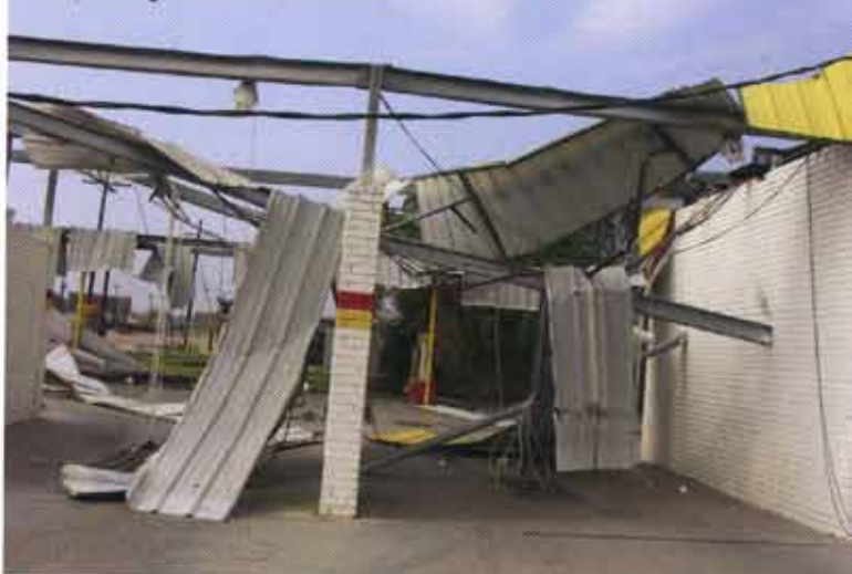
The bldg. structure in Bridge City wash bays mangled with wire and metal.
