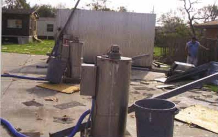
Side view of West Orange vac bay area where vac shed is totally blown away.
